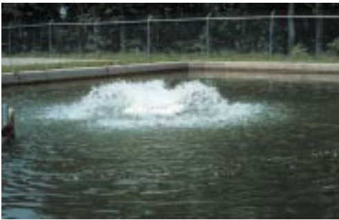
Fountain-like aerator draws water from underneath.
